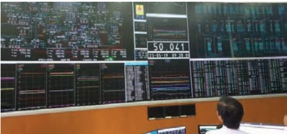
Gambar 1.14 SCADA Control Centre
