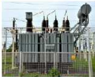
Transformator Step Up
